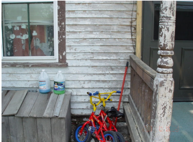
Older buildings with chipping paint pose significant lead poisoning hazards.
